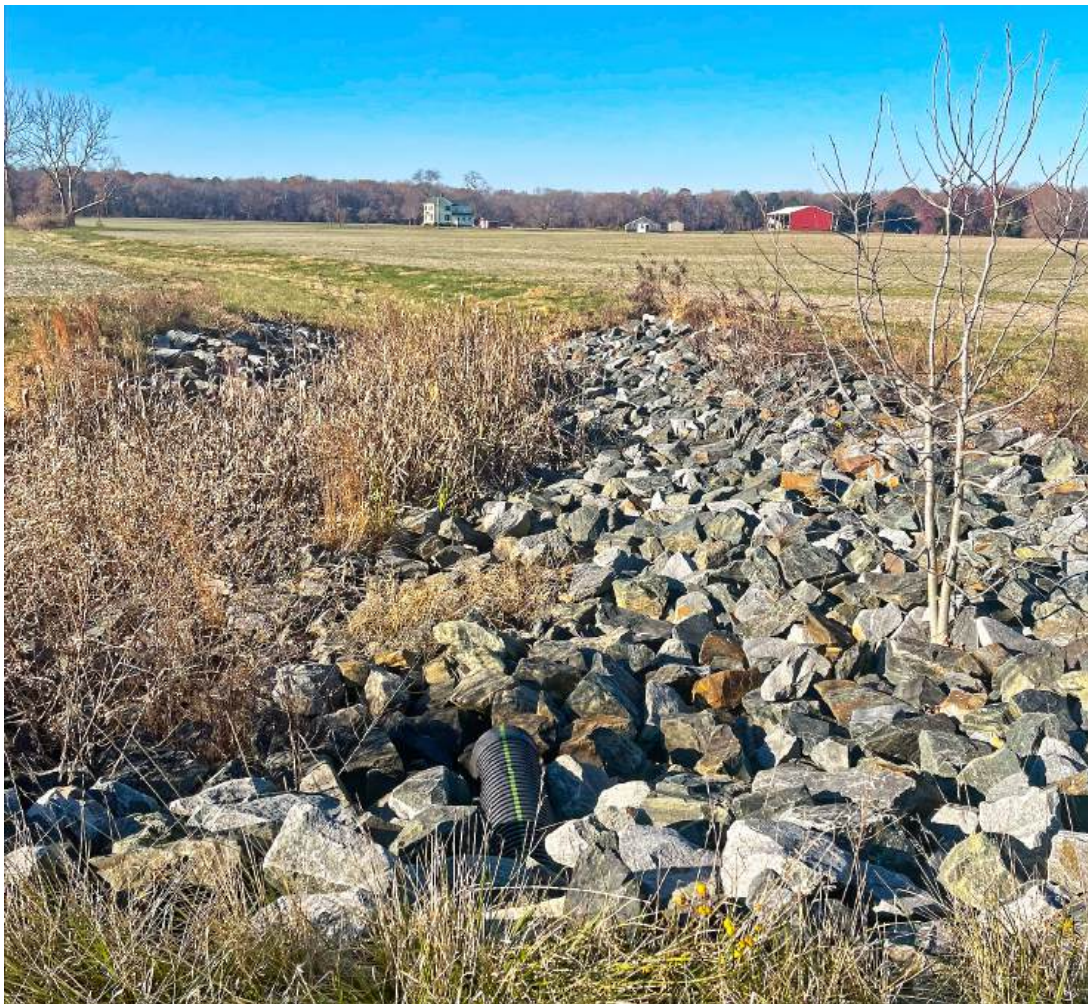
Drainage pond and stone spillway, Kingston Landing Photo: Will Beaven
